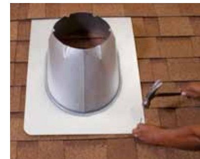
11. Slip the flashing over the roof hole so the top edge is under the shingles above. Nail the flashing to the roof across the top and down 1/2 each side. Seal flashing and nailheads with weatherizing sealant.
